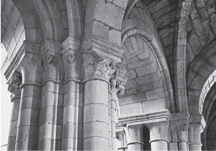
Fig. 25. Santa María de Gradefes, ambulatory viewed from northeast chapel, first two hemicycle piers on the north side, c. 1177-1190s. (photo: author)
