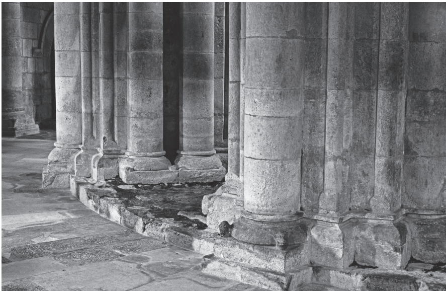
Fig. 26. Santa María de Gradefes, plinths and lower courses of hemicycle piers in front of southeast chapel, c. 1177-1190s. (photo: author)
